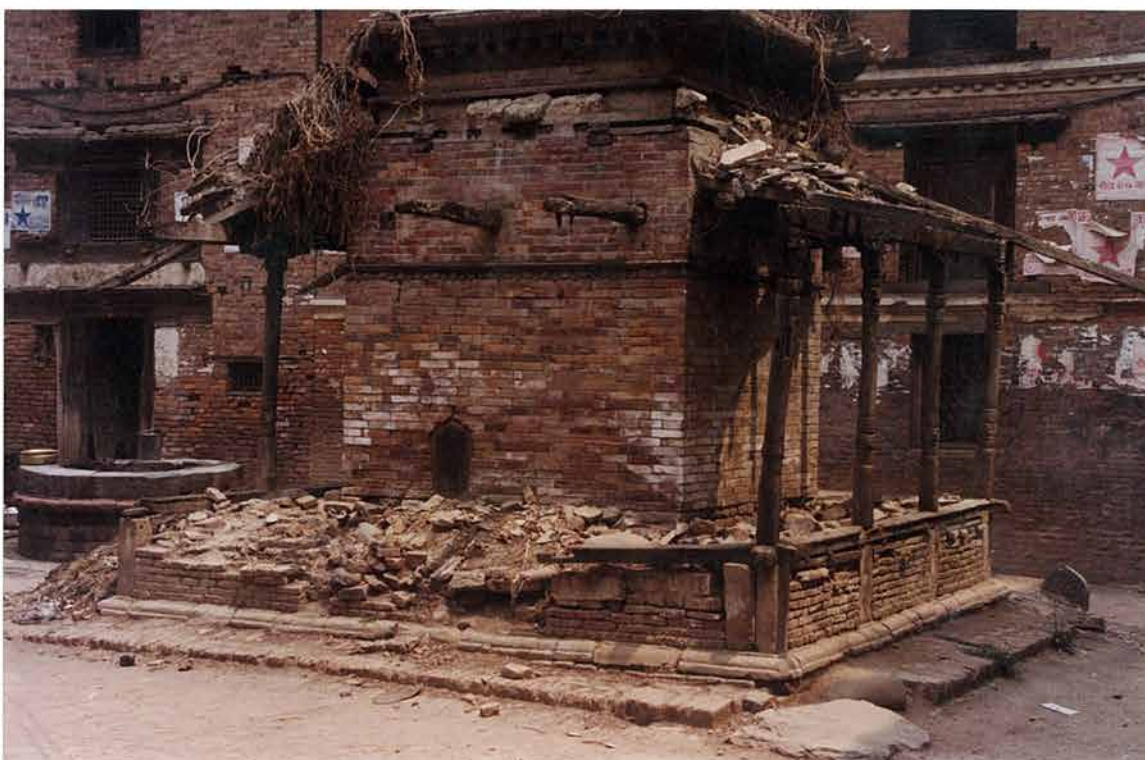
Below: most of the plinth planking is lost. On the south elevation base stones for the two middle timber posts were also lost. Photo December 1997.
