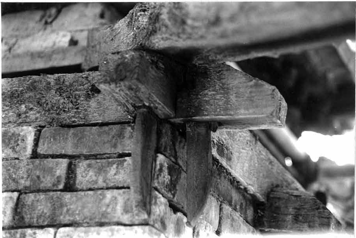
Corner lap joint of outer wall plate on middle level damaged by exposure to weather.
