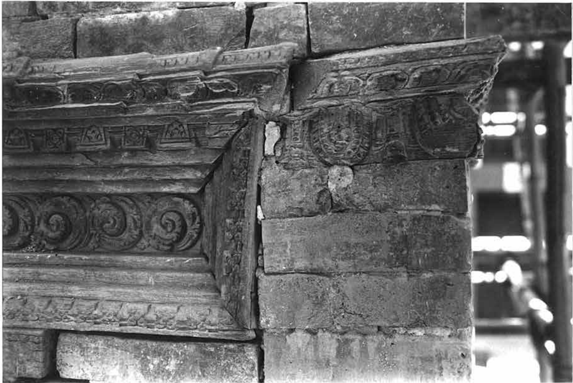
Existing lintel of the door frame on the ground floor level. The edge of the masonry wall is 2" longer on the left side leaving a space between the extended door lintel and timber cornice that is filled by a piece of brick.
