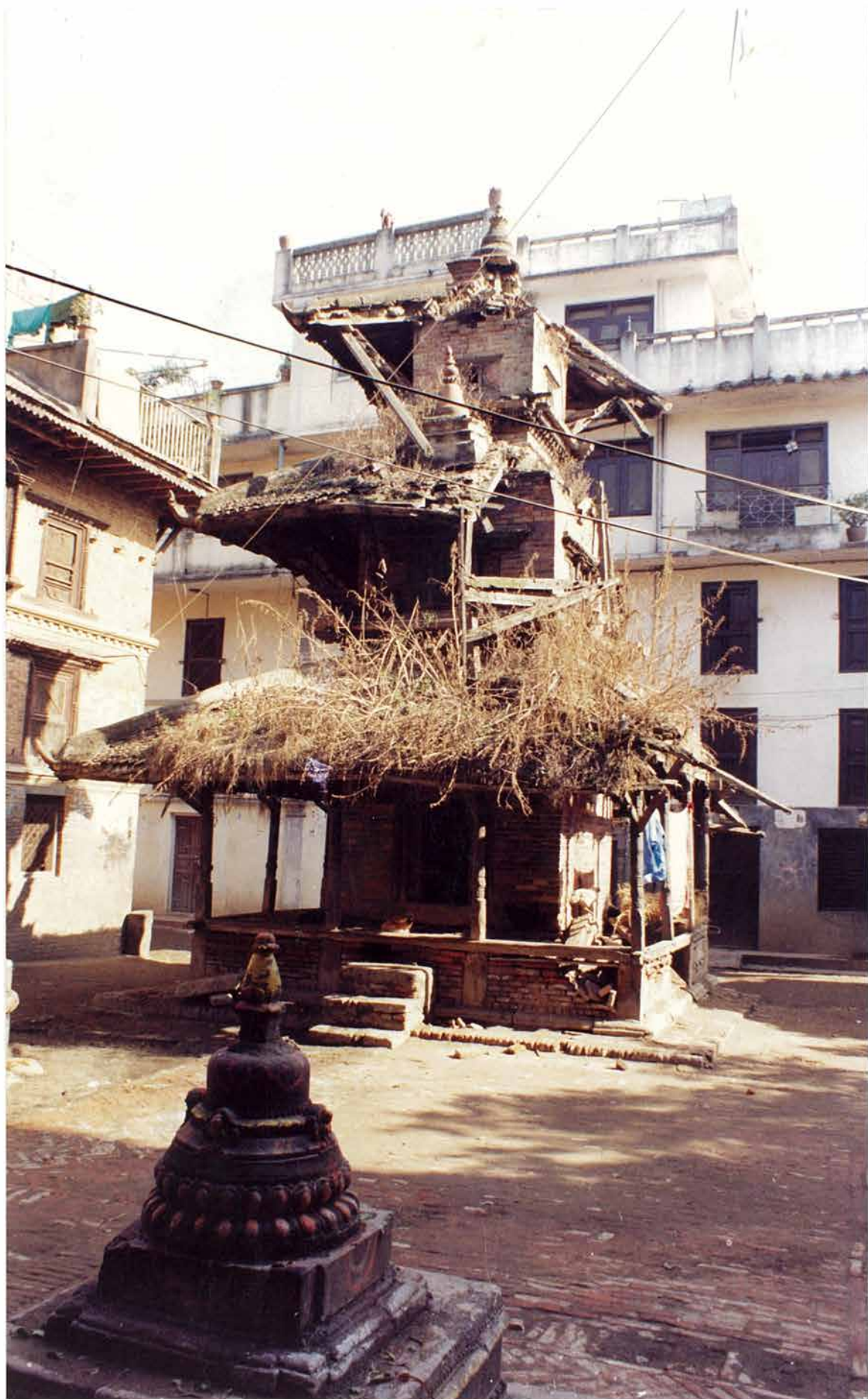
Roof largely collapsed. Seen from west. Photo 1994
