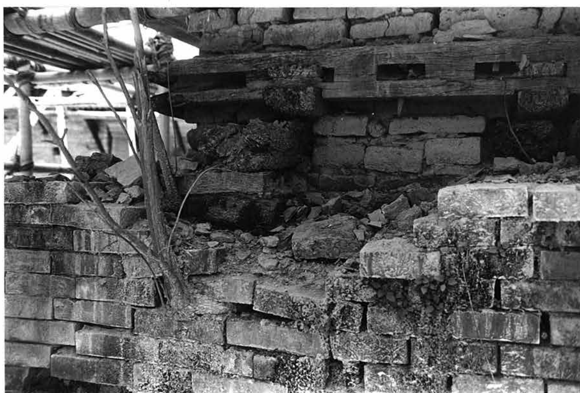
Above: water damage at middle level showing outer wall plate and washed out mud mortar at upper layers of brick.
