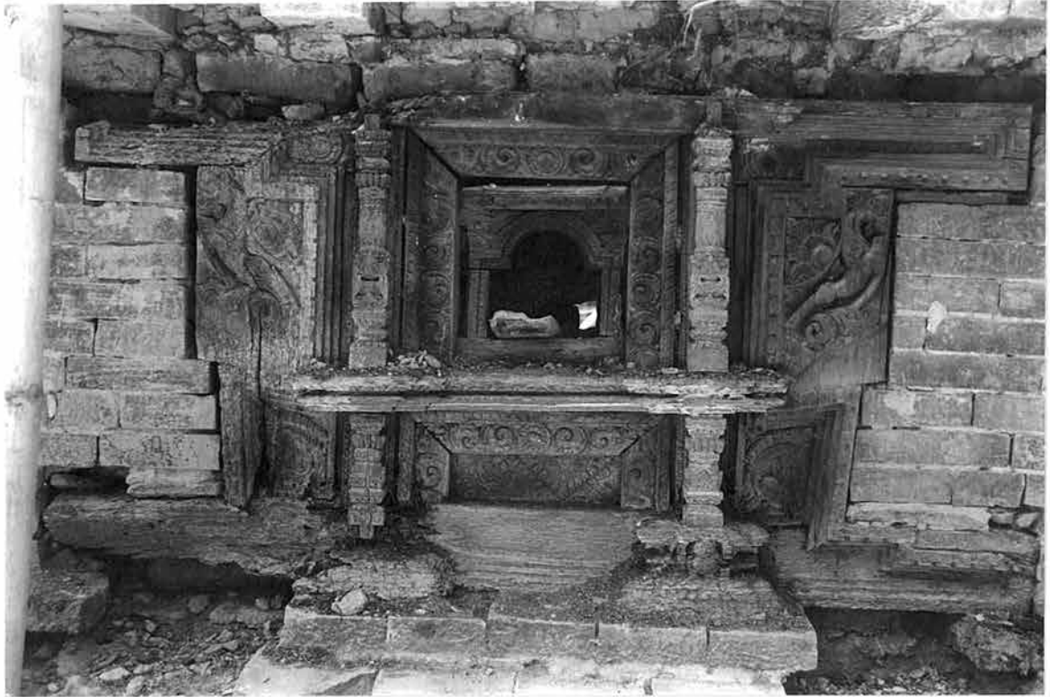
Existing Condition of Decorative Carved Window ( Gh jhyah ) PHOTO OF GH JHYAH AT EAST FACADE
