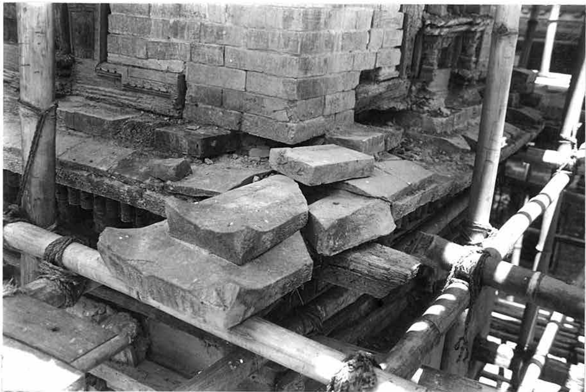
Top: completely missing lah kah and lah phvah at south-west corner.
